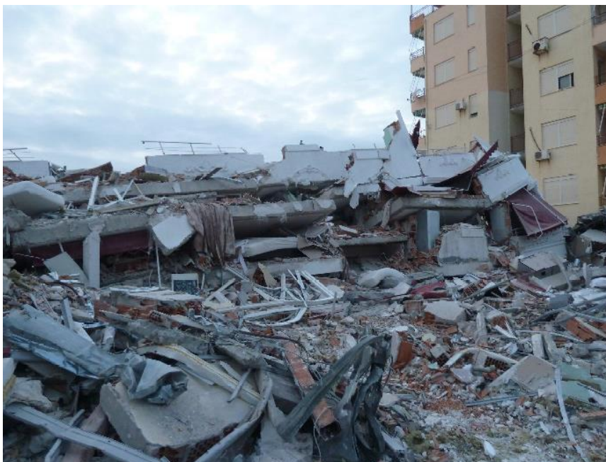
Slika 3. Popolnoma uničen hotel Mira Mare v Draču. (vir: https://www.emsc-csem.org/Files/news/Earthquakes_reports/Newsletter_15_2019_Albania_EQ.pdf ) Figure 3. Totally collapsed hotel Mira Mare in Durrës (Source: https://www.emsc-csem.org/Files/news/Earthquakes_reports/Newsletter_15_2019_Albania_EQ.pdf )
